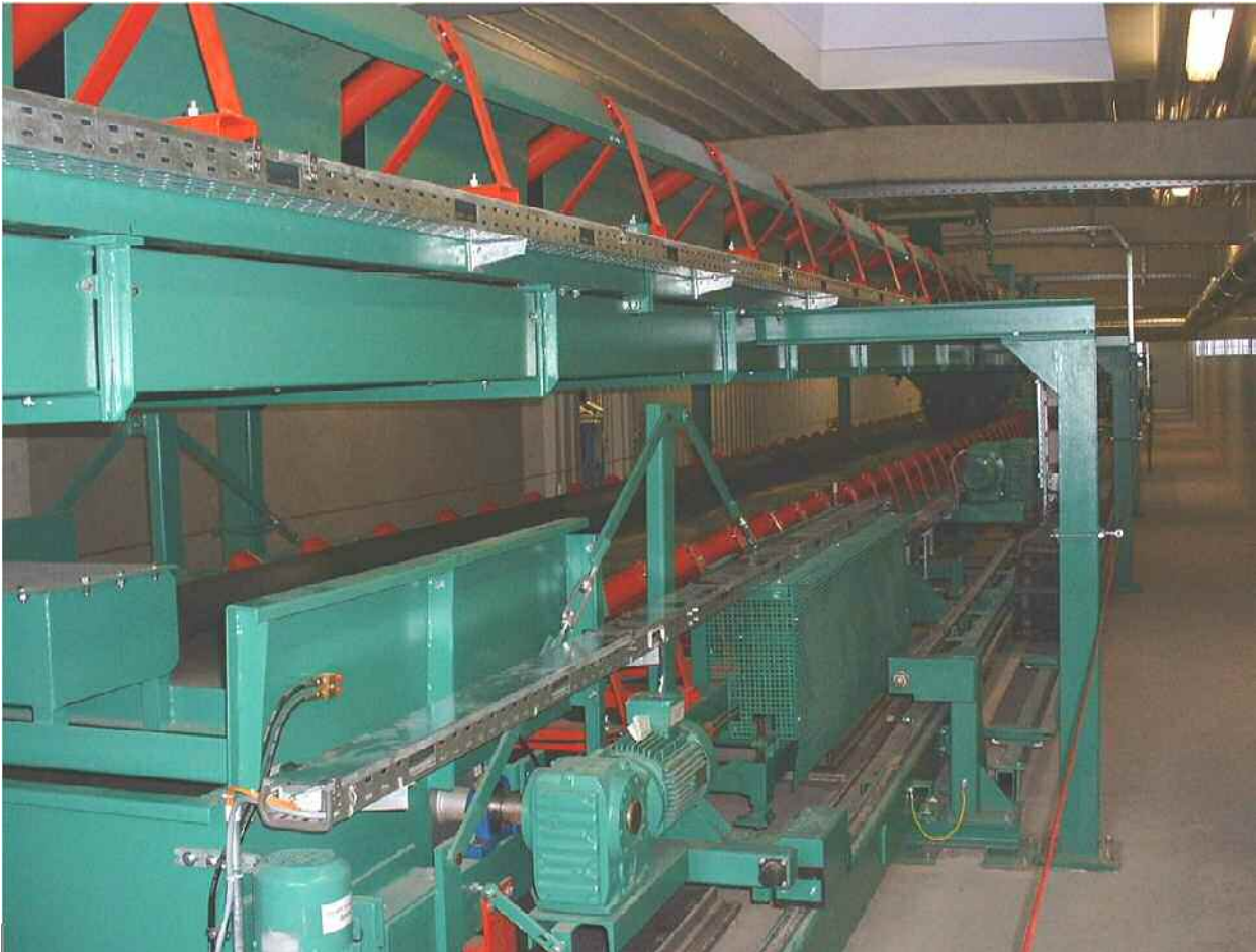
Figure 7 Conveyor System on the Roof of the Tunnel
