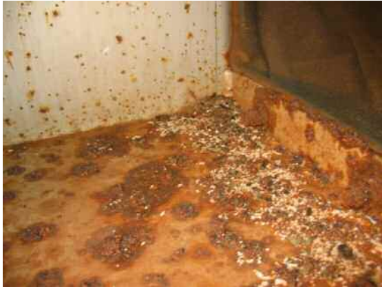
a) Dirty gas channel (pitting)
