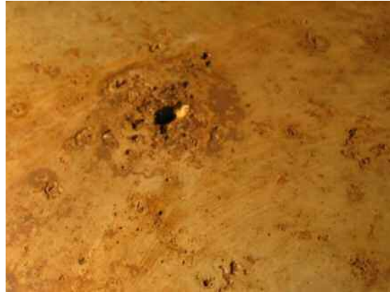
b) Pitting detail
