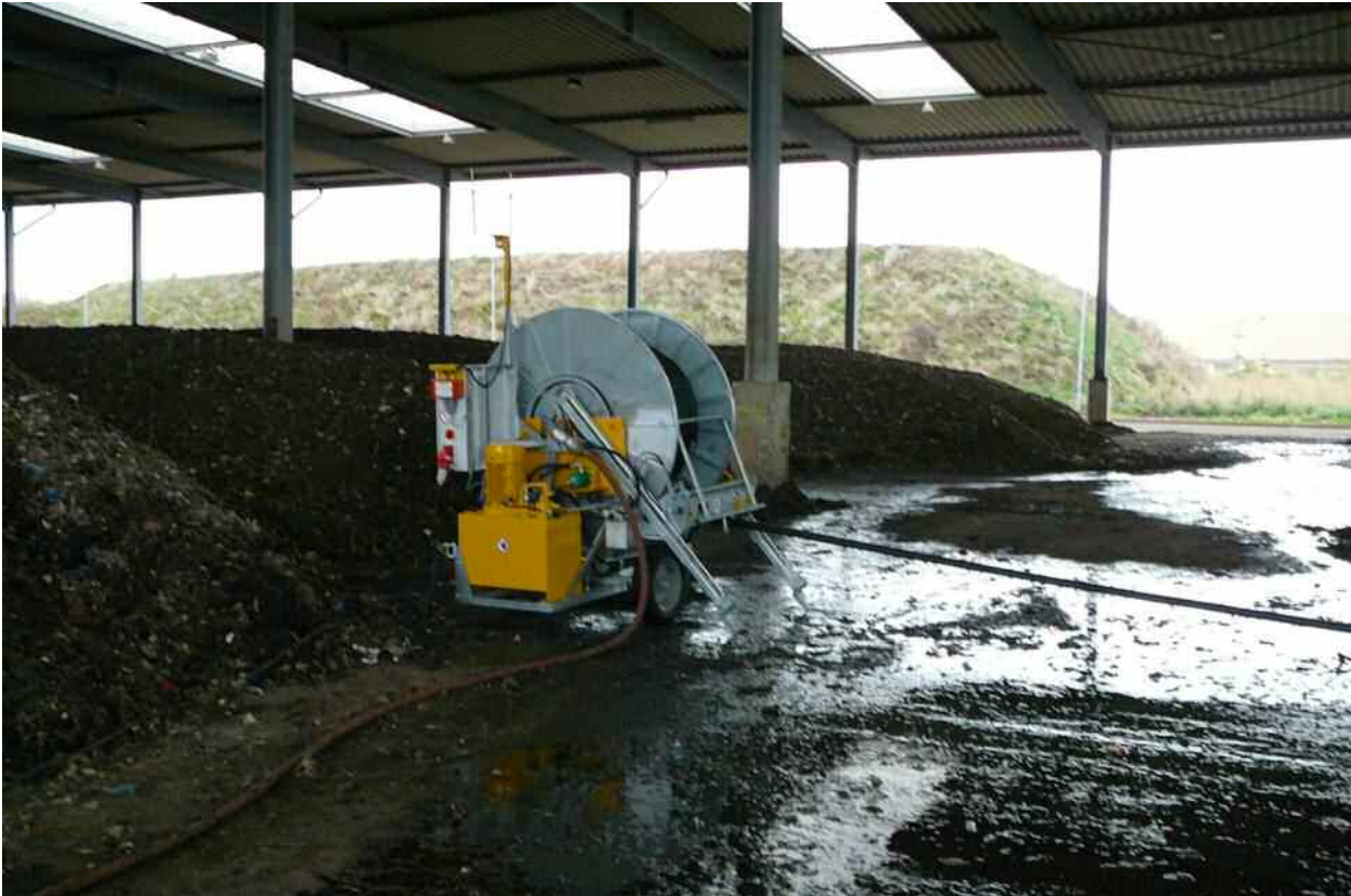
Figure 3: Maturation MBT Schwanebeck, irrigation unit
